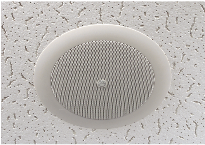
FAP40T (Shown Installed in Drop Tile Ceiling)
